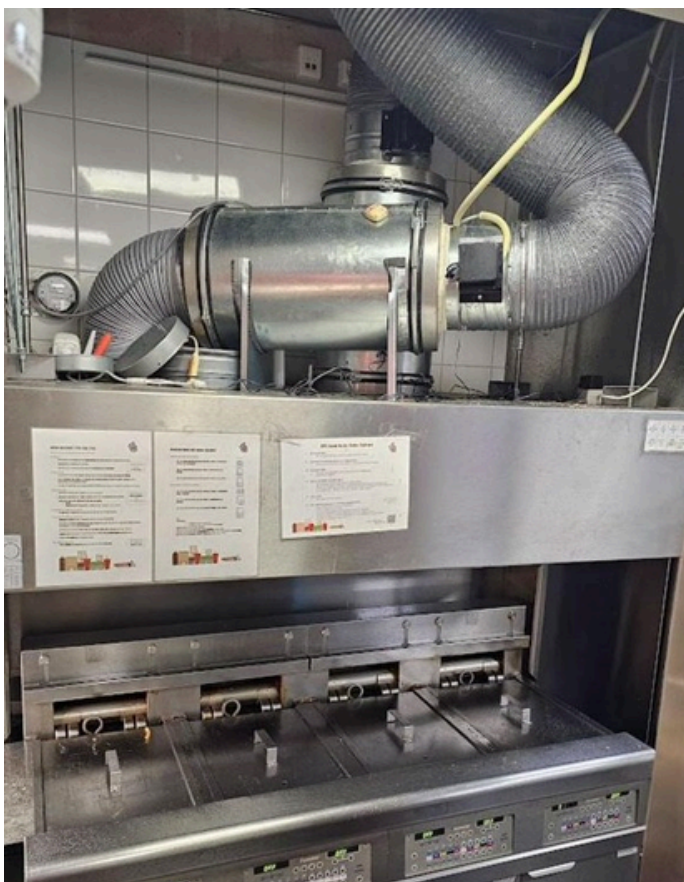
Horisontal Lynx Kitchen installation.
